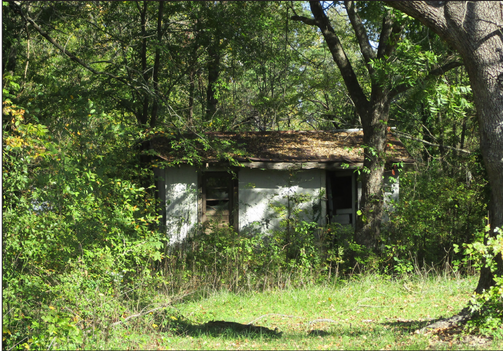
Photograph 9: South elevation of the shed in the northwest corner of the property, looking north. (2016)
